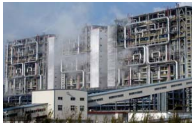
17 Siemens Gasifiers in Ningxia, China
